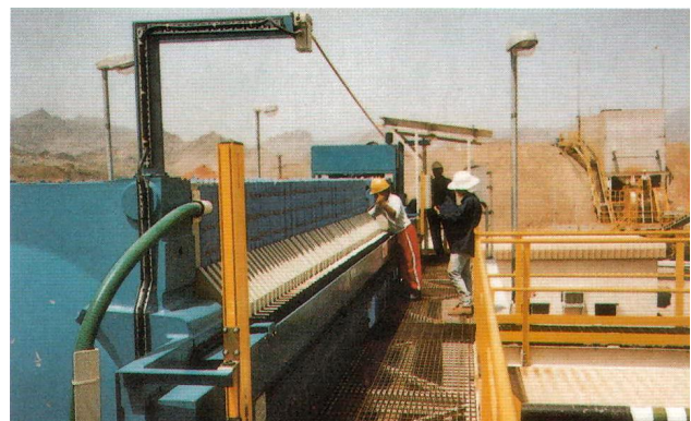
Refurbished press in operation
